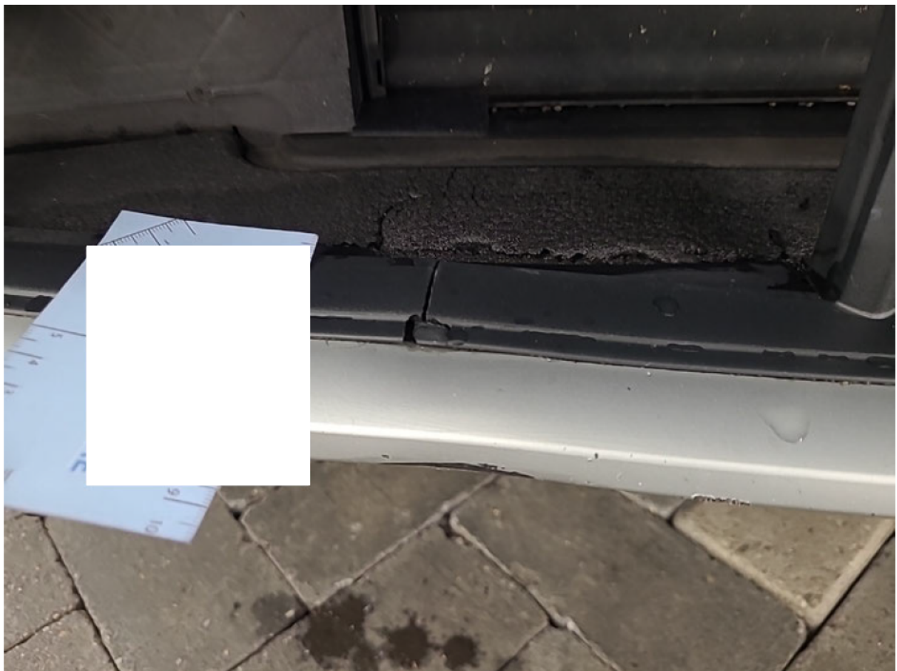
Damage photograph 12 of 32
