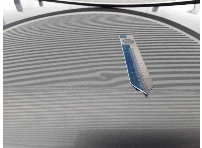
Damage 4: Roof: Roof - dent(s) - Smooth repair work
