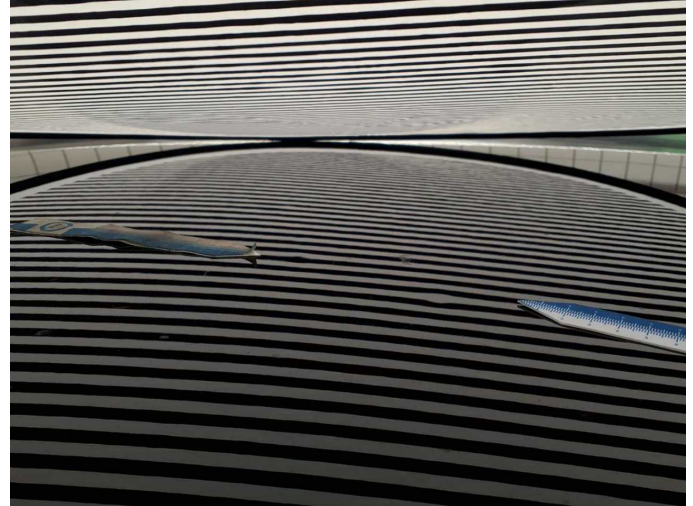
Damage 3: Roof: Roof - dent(s) - Smooth repair work
