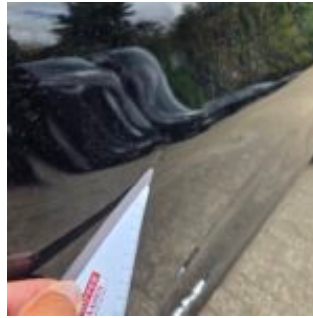
Repair Type Acceptable
