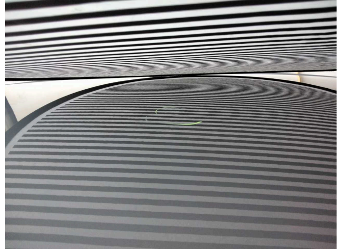
Damage 3: Roof: Roof - dent(s) - Smooth repair work
