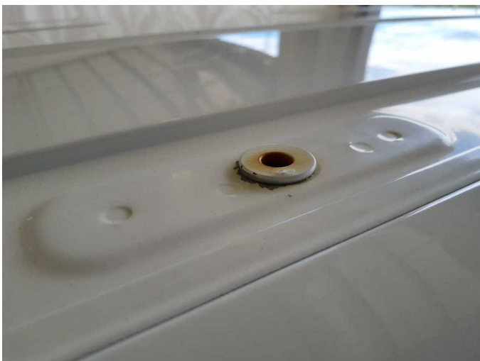
Damage 12: Roof: Roof (Korrosionsbildung) - Scratched - Paint
