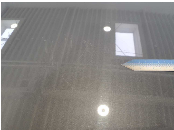
Damage 7: Roof: Roof - Scratch(es) - Paint
