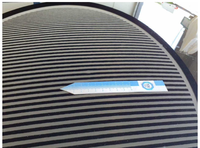
Damage 2: Roof: Roof - dent(s) - Smooth repair work
