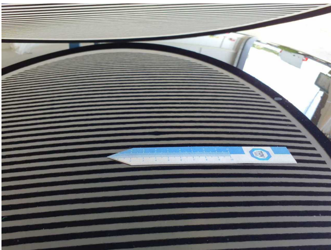
Damage 2: Roof: Roof - dent(s) - Smooth repair work
