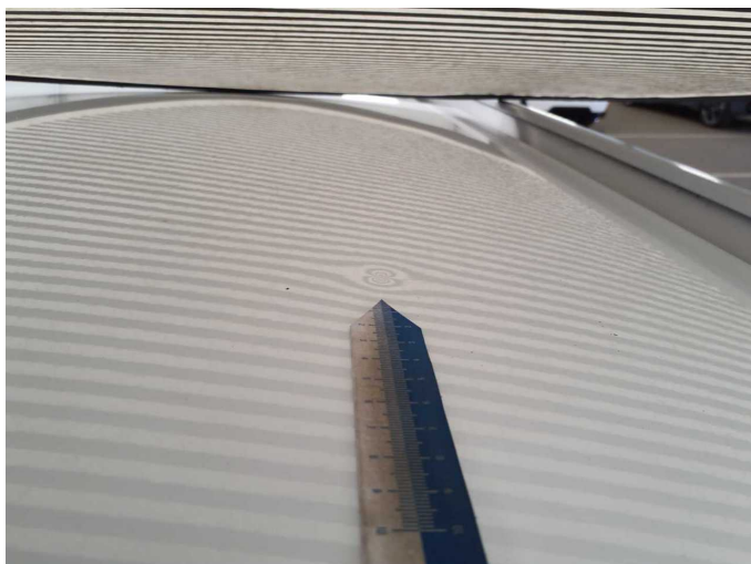
Damage 5: Roof: Roof - dent(s) - Smart repair
