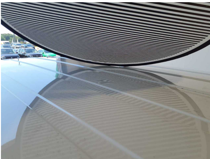
Damage 6: Roof: Roof - dent(s) - Repair and paint
