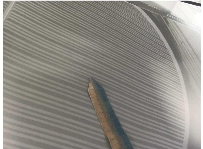
Damage 4: Roof: Roof - dent(s) - Smooth repair work
