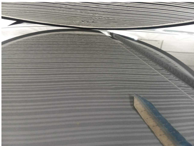
Damage 4: Roof: Roof - dent(s) - Smooth repair work
