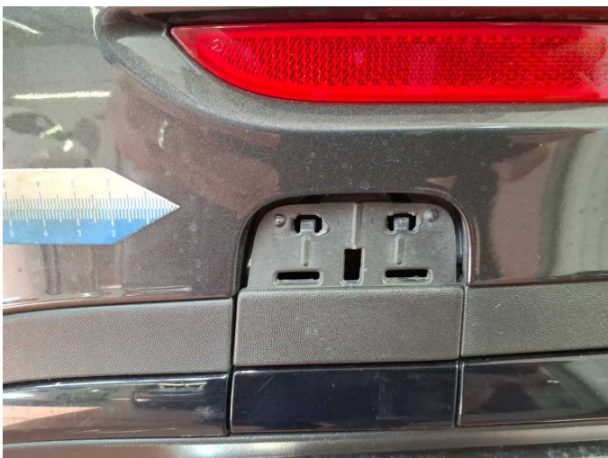
Missing part 1: Equipment: Towing eye (Lackierte Abdeckung) - Missing - Replace
