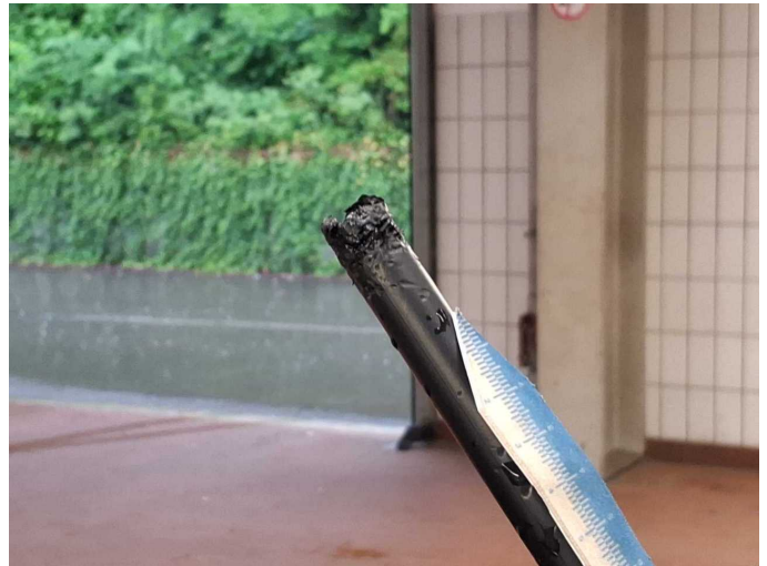
Damage 4: Roof: Stub aerial - Damage caused by marten / rodent - Replace
