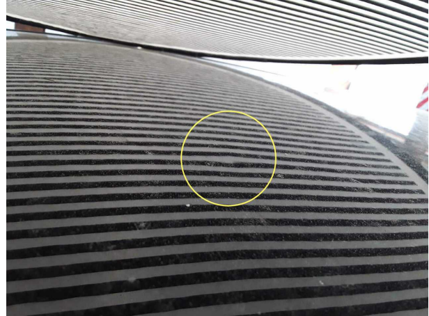
Damage #4: Roof: Roof - dent(s) - Smooth repair work
