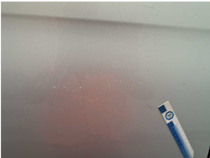
Damage 7: Sliding door, right: Sliding door - Dent / paintcoat damage - Repair and paint
