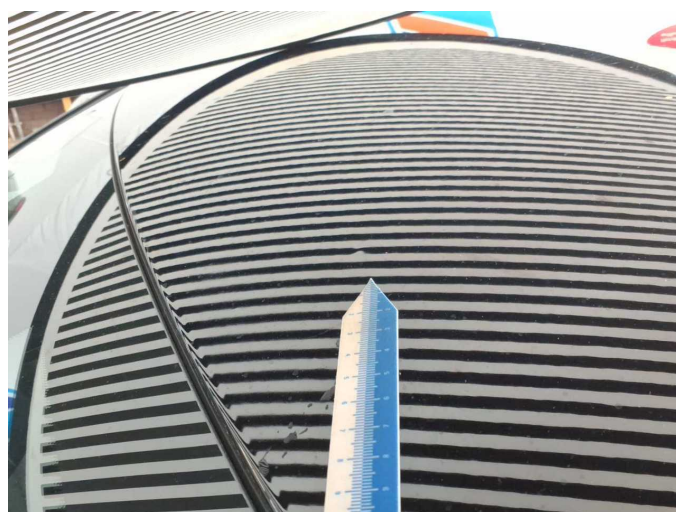
Damage 1: Roof: Roof - dent(s) - Smooth repair work
