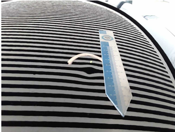
Damage 4: Roof: Roof - Damage by hail - Repair
