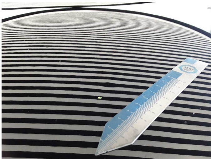
Damage 4: Roof: Roof - Damage by hail - Repair
