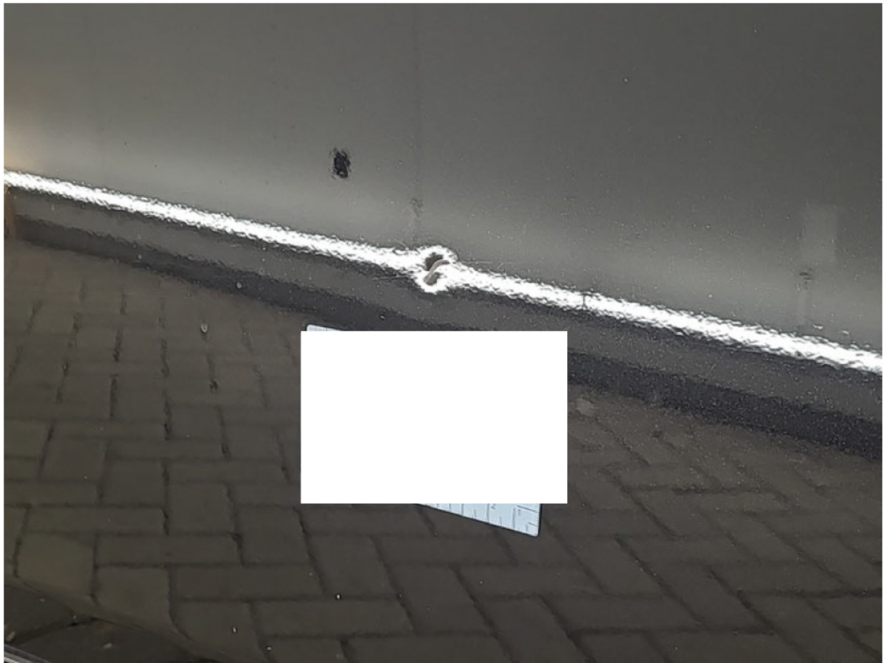
Damage photograph 9 of 30
