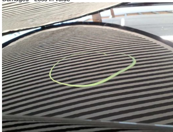
Damage #4: Roof: Roof - dent(s) - Smooth repair work
