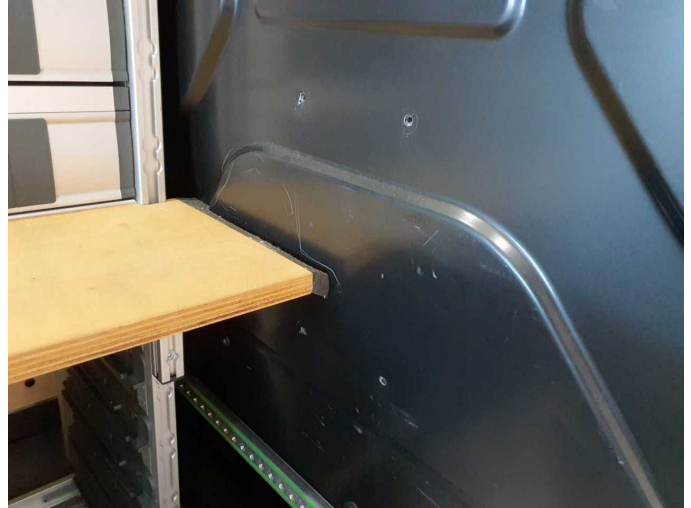
Damage 7: Body: Partition wall - Holes - Replace
