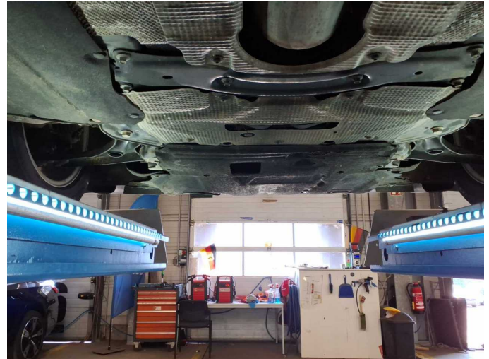
Damage 4: Gearbox: Gearbox - Leaking - Perform diagnosis
