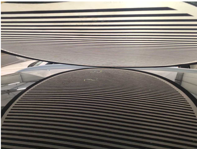
Damage 10: Roof: Roof - dent(s) - Smooth repair work
