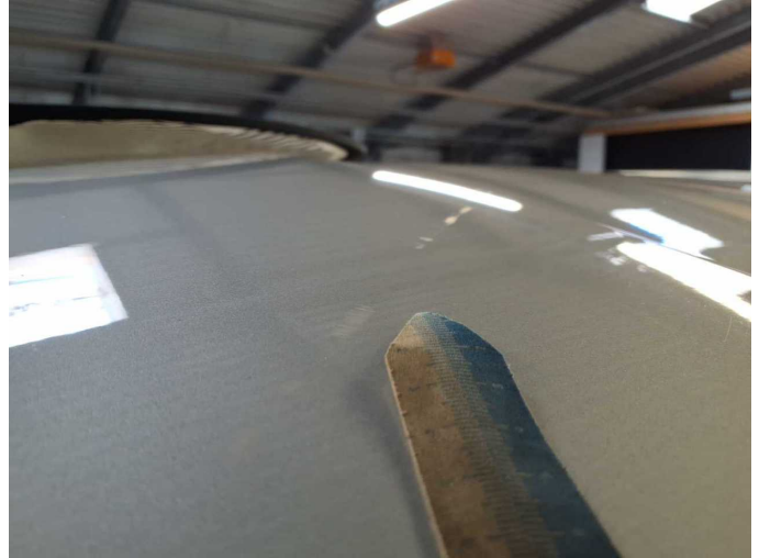
Damage 11: Roof: Roof - Scratch(es) - Paint
