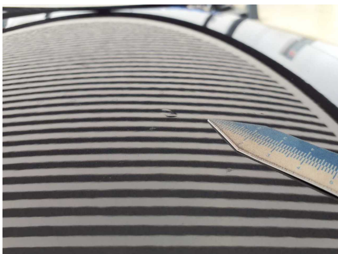
Damage 12: Roof: Roof (Anätzung) - Paint defect - Repair and paint
