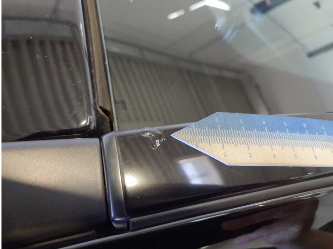
Damage 1: Roof: Cowl - right side - Corrosion - Replace
