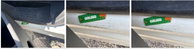
Wheel cover RL, Missing, Replace
