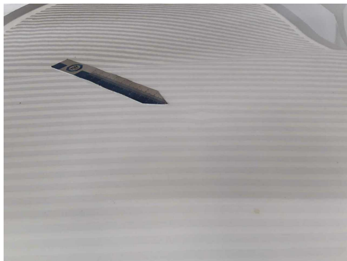
Damage 5: Roof: Roof - dent(s) - Smooth repair work
