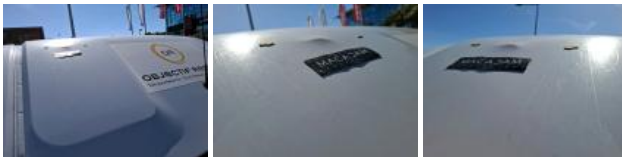
Roof, cabin, Dent(s), Repair and paint (complete)
