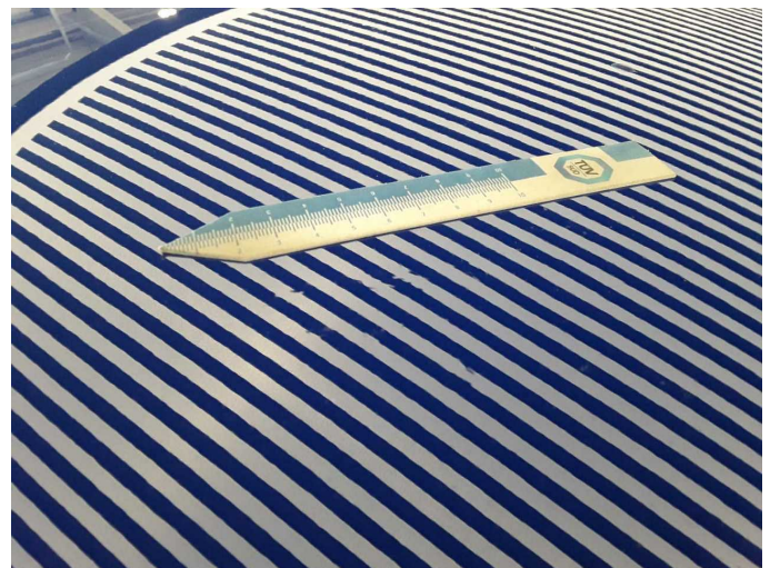
Damage 5: Roof: Roof (Anätzung) - Dent / paintcoat damage - repair according to calculation
