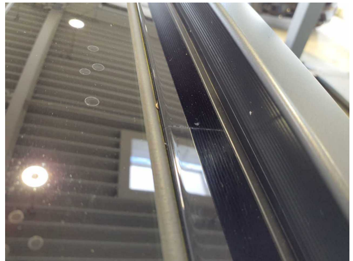
Damage 5: Roof: Cowl - left side - Broken / torn - Replace
