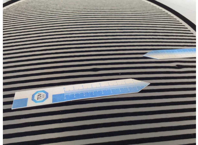
Damage 1: Roof: Roof - dent(s) - Smooth repair work
