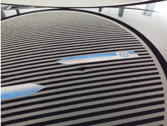
Damage 1: Roof: Roof - dent(s) - Smooth repair work
