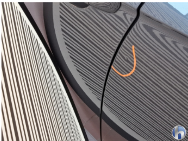
1. Tür Hinten - Links 1 Delle - Sanft Instandsetzen
