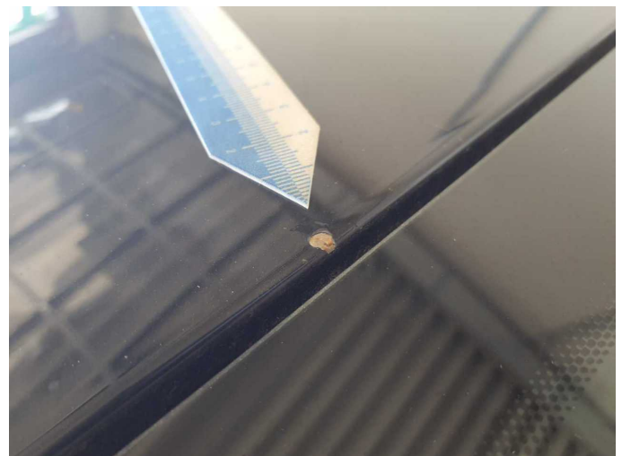
Damage 10: Roof: Roof - Corrosion - Repair and paint
