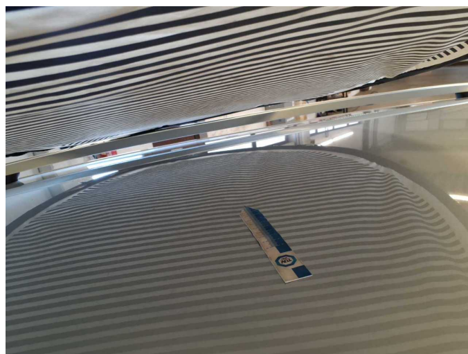
Damage 6: Roof: Roof - dent(s) - Smooth repair work
