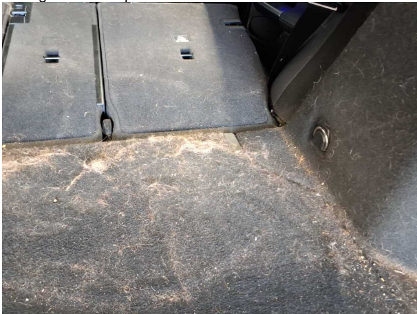
Damage #8: Interior: Interior - Soiled - Clean
