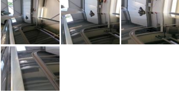
Roof, Hail damage, Paintless dent repair (hail)
