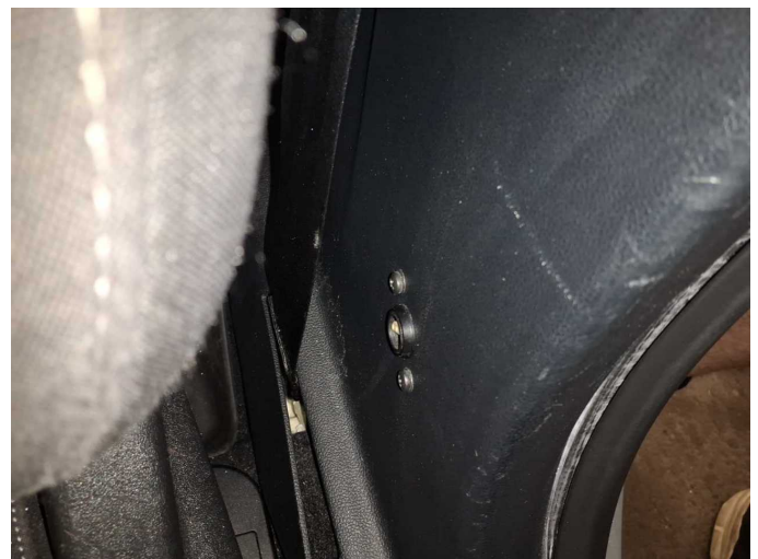
Damage 5: Trim / covers: B-pillar - trim - interior, left side (Fehlbohrungen) - Differs from the original configuration - Replace
