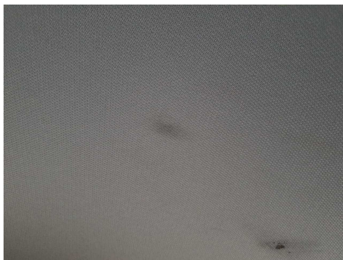
Damage 6: Trim / covers: Roof lining - Holes - Replace
