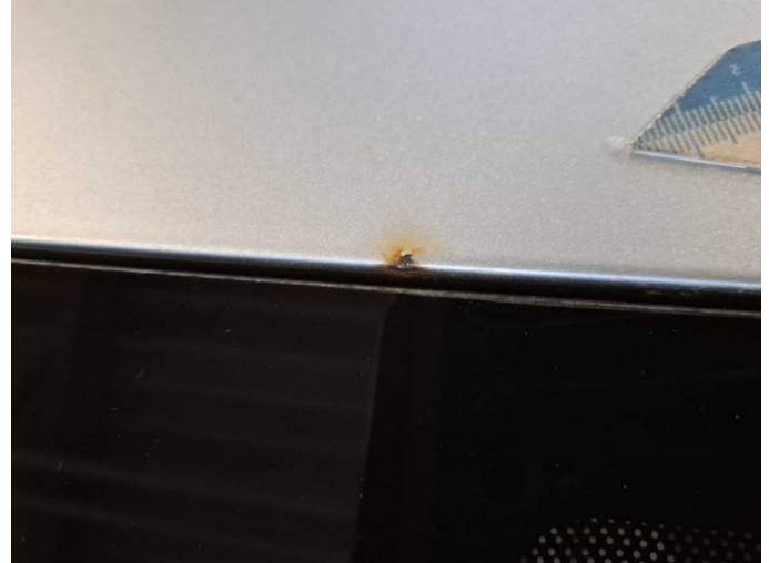
Damage 4: Roof: Roof - Corrosion - Smart repair
