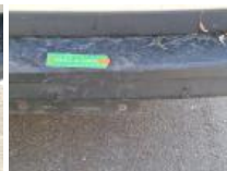
Reflector, Broken, Replace
