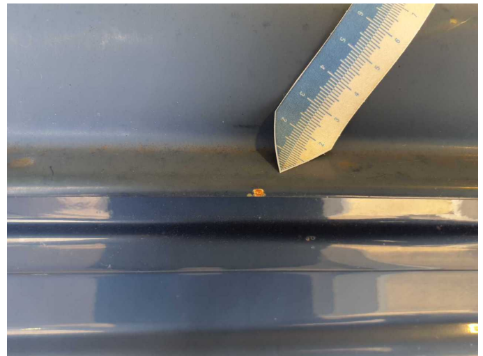
Damage 4: Roof: Roof (Dachkante) - Corrosion - Smart repair
