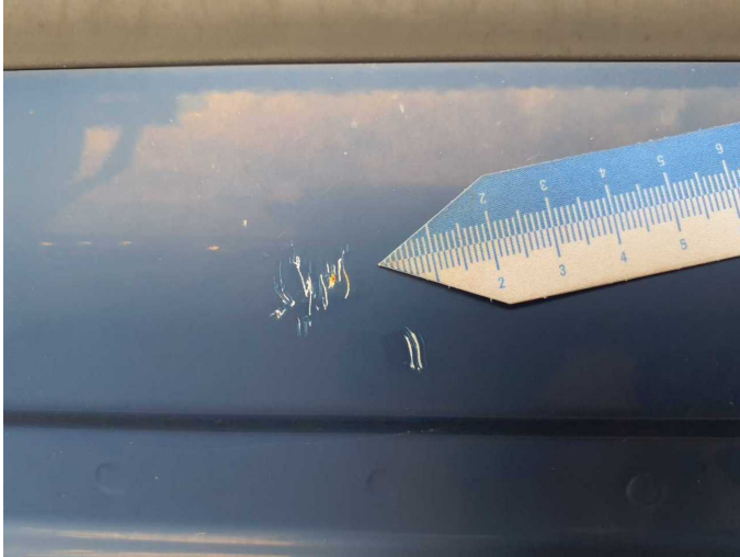
Damage 12: Cab: Rear panel - Corrosion - Repair and paint
