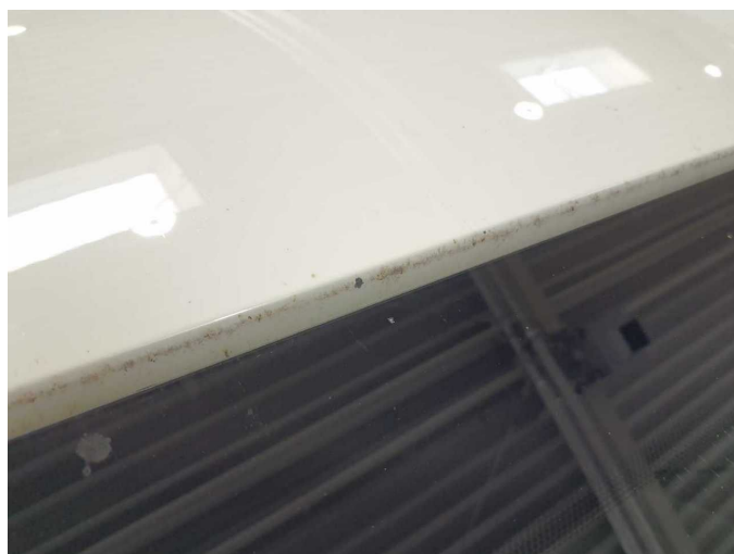
Damage 13: Roof: Roof (+ Kratzer, beginnende Korrosion) - Dent / paintcoat damage - Paint
