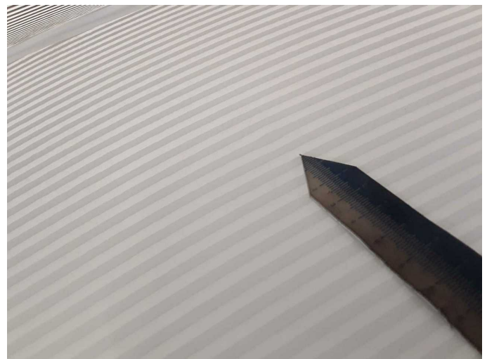
Damage 4: Roof: Roof (3 Dellen) - dent(s) - Smooth repair work
