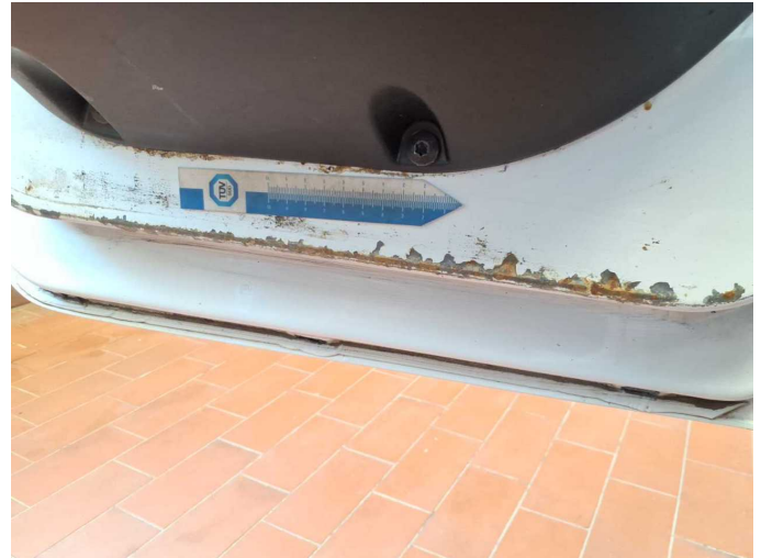
Damage 7: Door - front left side: Door (Unten / innen) - Corrosion - Loss in value
