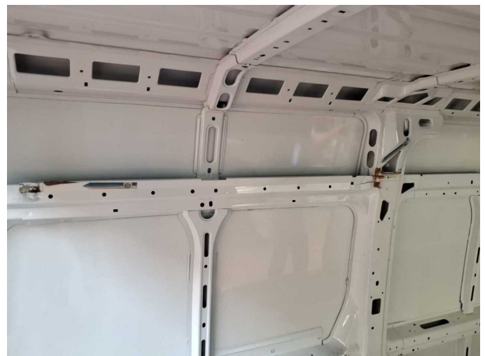
Damage 9: Side panel - rear left side: Side panel (Innen) - Corrosion - Smart repair
