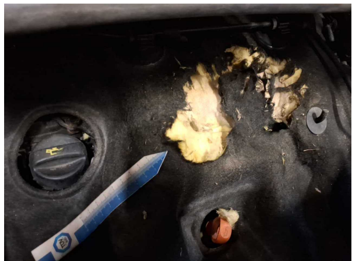
Damage 2: Engine: Engine cover (Isolierung Motor) - Damage caused by marten / rodent - Replace
