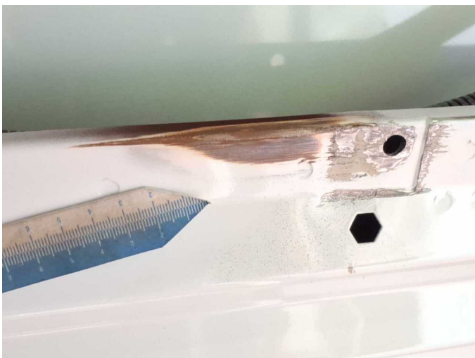
Damage 10: Side panel - rear right side: Side panel (Innen) - Corrosion - Smart repair
