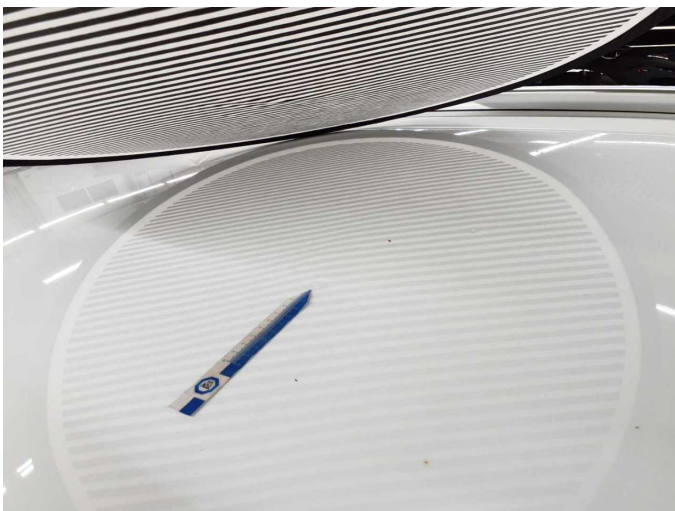
Damage 3: Roof: Roof - dent(s) - Smart repair
