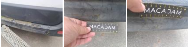
Rear bulkhead lining, Broken, Replace
