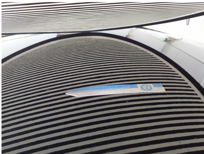
Damage 7: Roof: Roof - dent(s) - Smooth repair work
