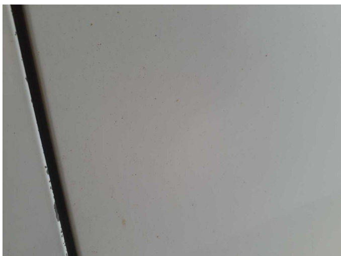
Damage 4: Body: Body (Flugrost) - Soiled - Conditioning
