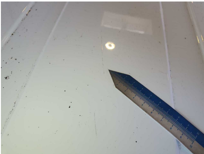
Damage 7: Roof: Roof - Scratch(es) - Paint
