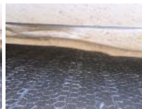
Step R, Broken, Acceptable
